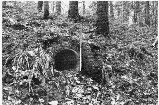
Ashburnham OB emergency exit tunnel with single course of brickwork still in place
